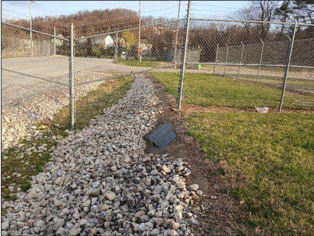
Photo looking north at exposed HDPE liner on the east side of the GATE 5 access road.
