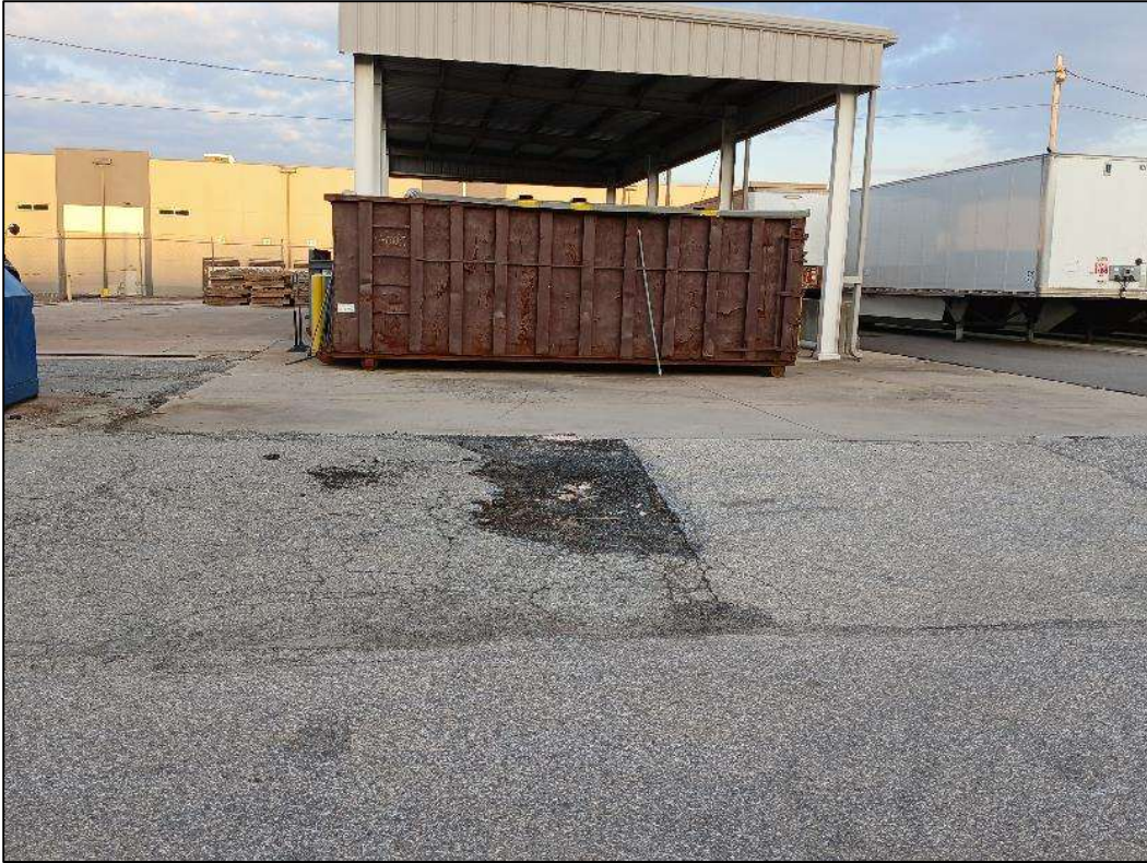
Photo looking west at distressed asphalt east of the roll off box lean-to structure.
