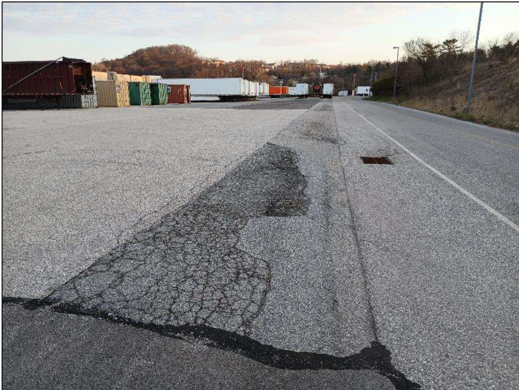
Photo looking north at distressed asphalt east of the safety shed.
