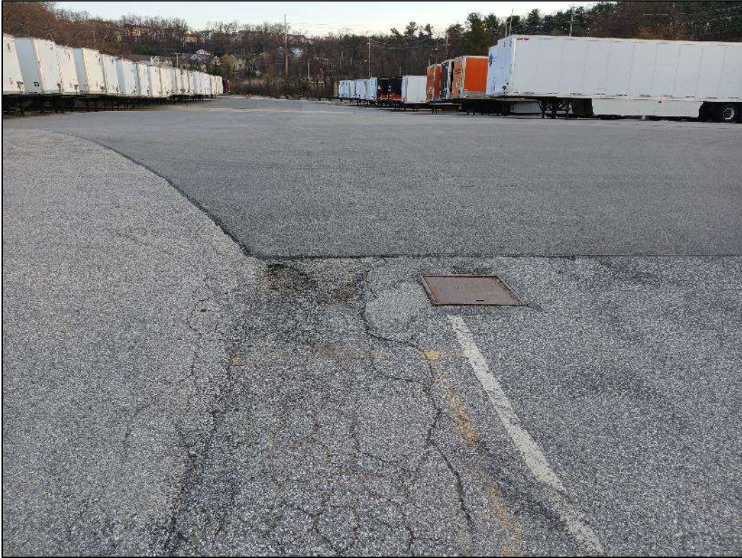
Photo looking north at distressed asphalt in the intersection near the fire pond.
