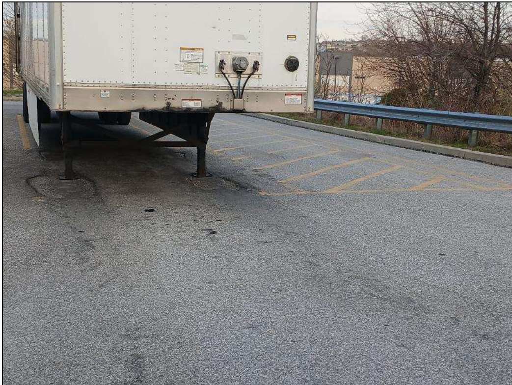
Photo looking west at distressed asphalt south of the fire water pond.
